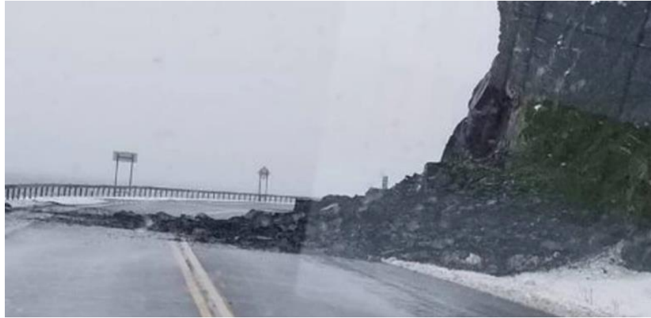
Figure 25. Rockfall that occurred 16 April 2019 obstructing Route 132. © Philippe Langlais, TVA Nouvelles
